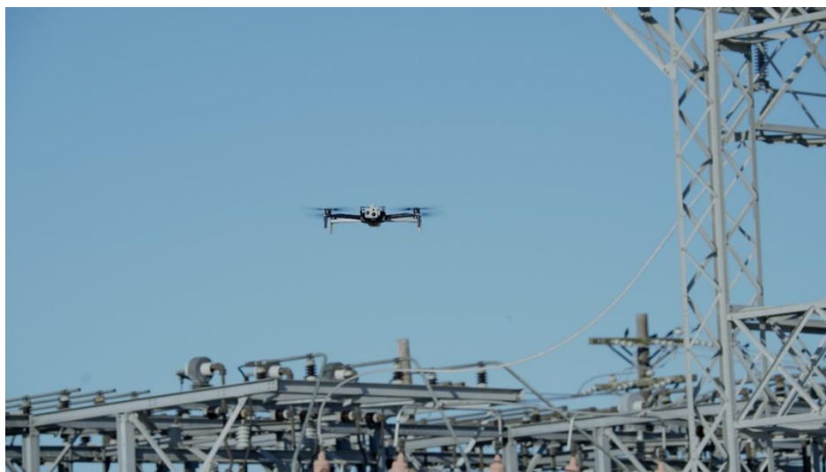
Above: A Skydio X10 performing autonomous routine inspection of an electric substation.
